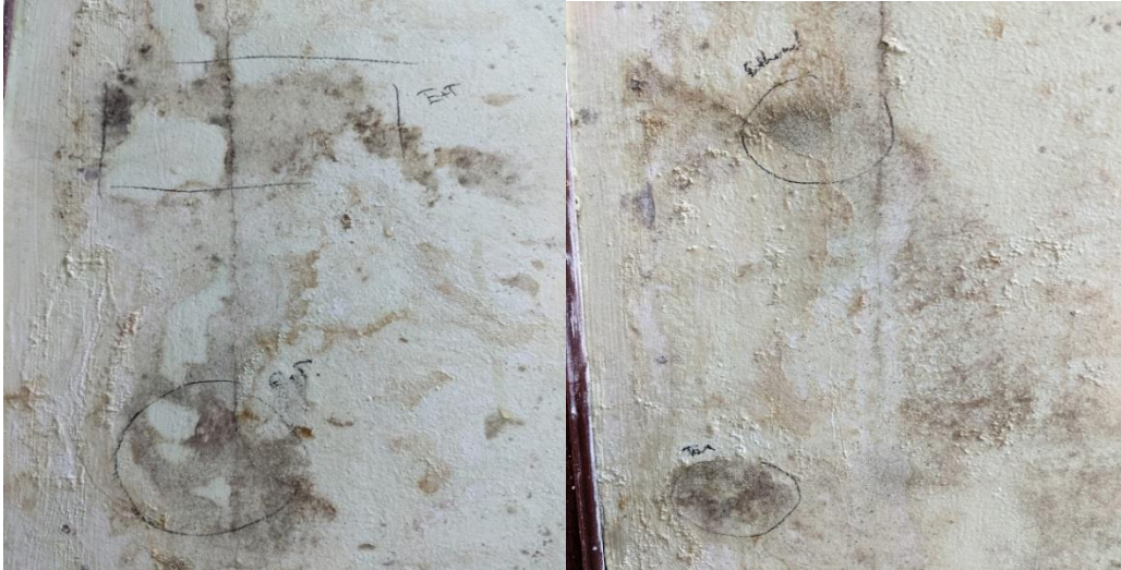
Figure 1. Mold growth and destruction of paint on walls, and mold sampling locations.
