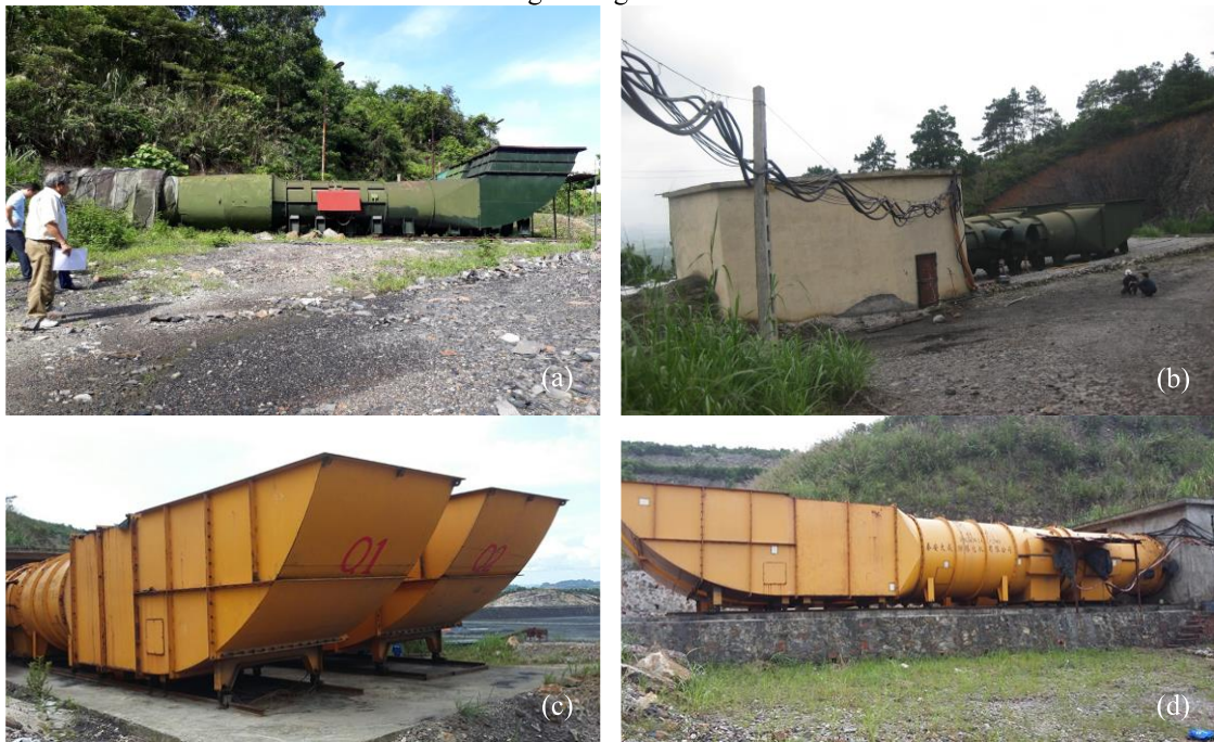
Figure 2. Main fan station - Design II: (a) FBDCZ-II-No.18 at North Mong Duong, Mong Duong coal mine; (b) FBDCZ-No.20 at Hong Thai coal mine; (c-d) FBDCZ-8-No.24/2x280 at Ha Lam coal mine
