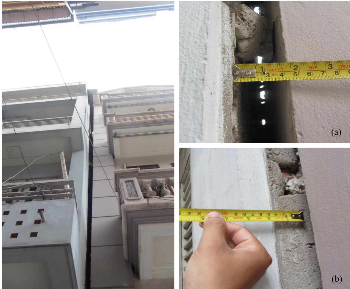
Figure 15. Subsidence between House number 130 and 131 in Vinh Hung Ward, Hoang Mai District: (a) Separation in horizontal direction, (b) deviation in depth of the houses
