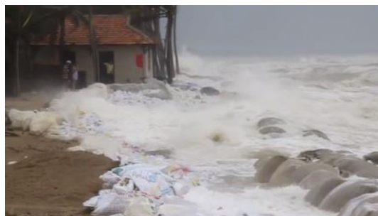
c) Large waves destroyed the revetment at the main Cua Dai beach [Photo taken on 18 October 2016]
