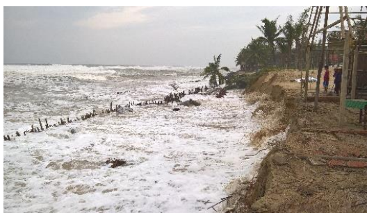
b) Large waves caused coastline erosion at Tan My beach [Photo taken on 18 October 2016]
