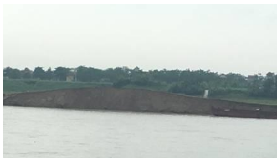
Fig. 6. Slump on the left bank of Red river in Me Linh, Hanoi
